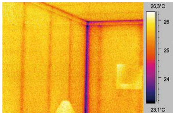
IR image taken from inside. The skeleton frame is visible, as well as the screws fixing the panelling to the frame. The corner is much colder, though such "corner effects" are normal. Source: FLIR©
