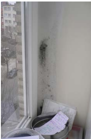
Mildew in a cold area
