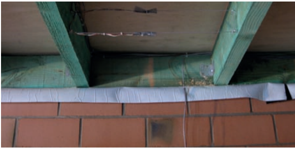
Installation of a membrane in the case of beams resting on the masonry (illustration, magazine CSTC -Contact nr. 33 (2012)
