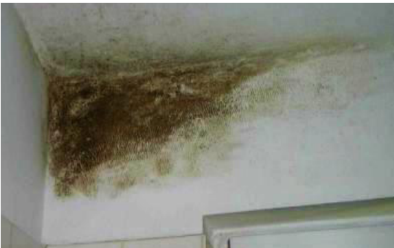
Example of mould related to a thermal bridge, (Rechtsanwalt Friedhelm Thome, Köln).
