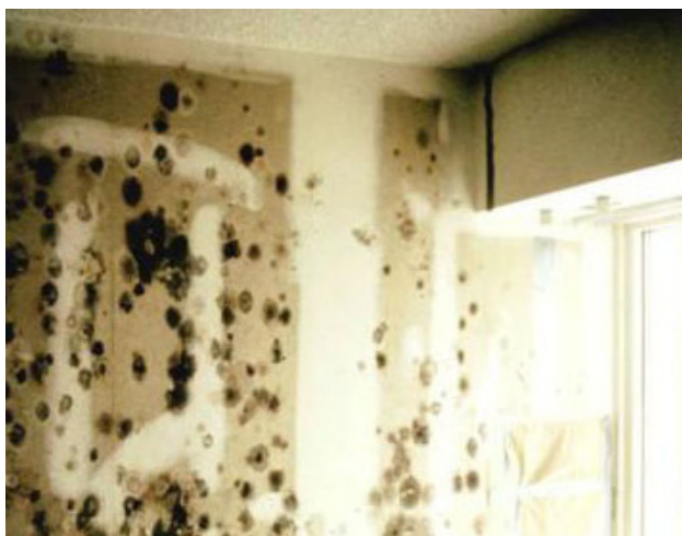
Example of mould due to inside condensation. ( Joe Lstiburek ).
